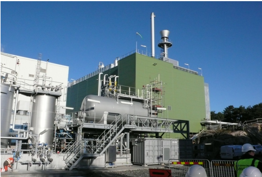
Figure 9. Photo of Gobigas plant before first gasifier startup (Oct. 2013). Reference: Göteborg Energi.
